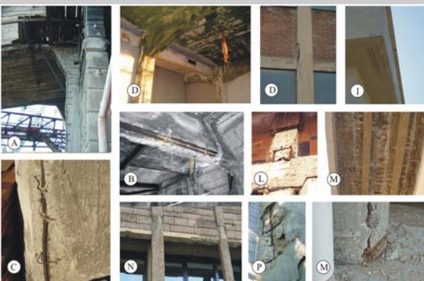
Figure 2 - Effects of corrosion (labels refer to the designation of the building according to Table 1).
